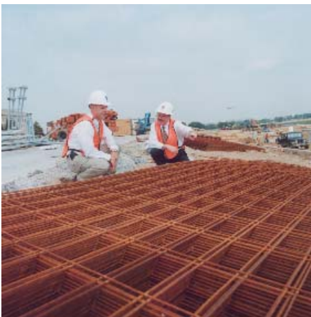
Evey (right) discusses progress on the Metro Entrance Facility work site with Brett Eaton, Information and Communications, Pentagon Renovation Program.
