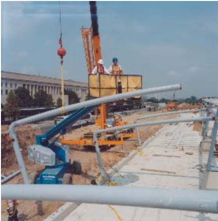
Evey (left) views progress at Metro Entrance Facility (MEF) work site from a cherry picker. With him is Fred Cobb, member of the MEF construction crew.
